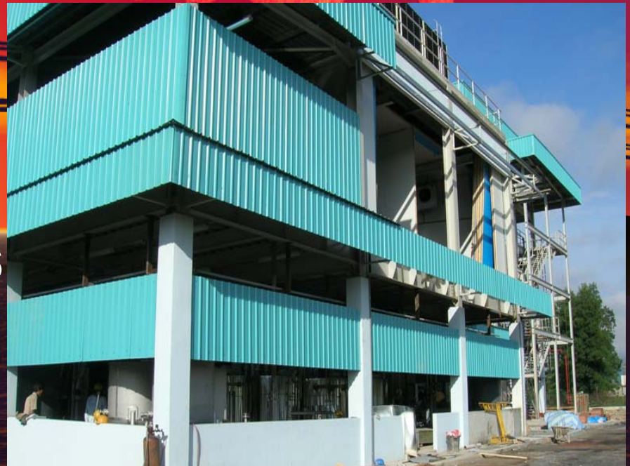
MPOB/Carotino 30,000 TPA Winter-grade PME Plant
